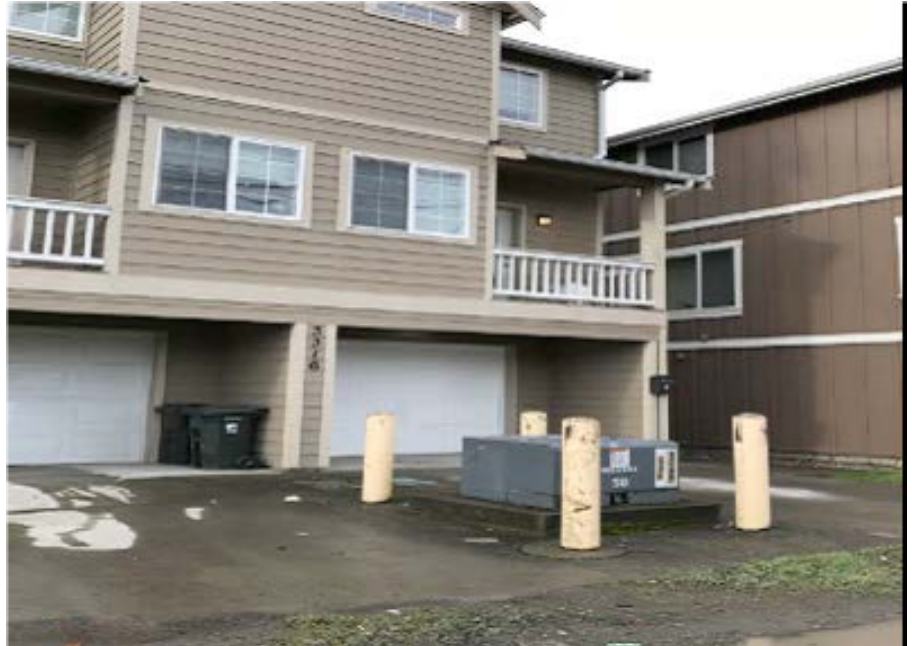
Photo US-7. This electrical box visually overpowers the townhouse.
