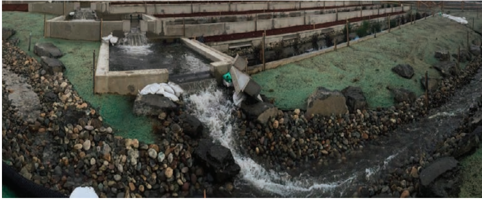
Photo E-3. Regional stormwater treatment facility (Pt Defiance Park).
