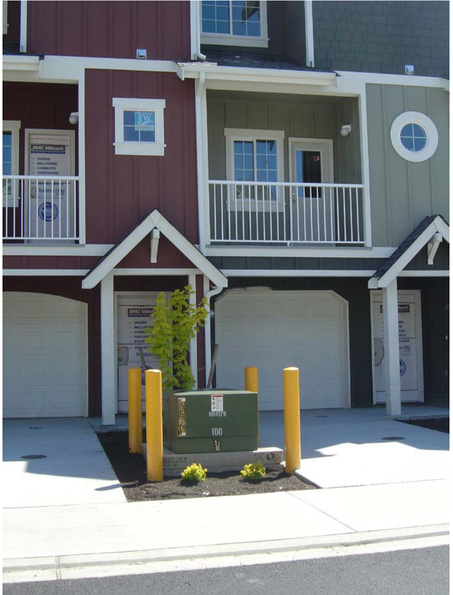
Photo US-4. An example of an overly conspicuous utility feature.
