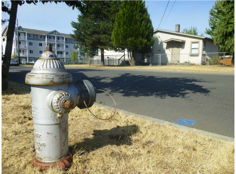
Photo US-2. Water hydrant, Madison District.
