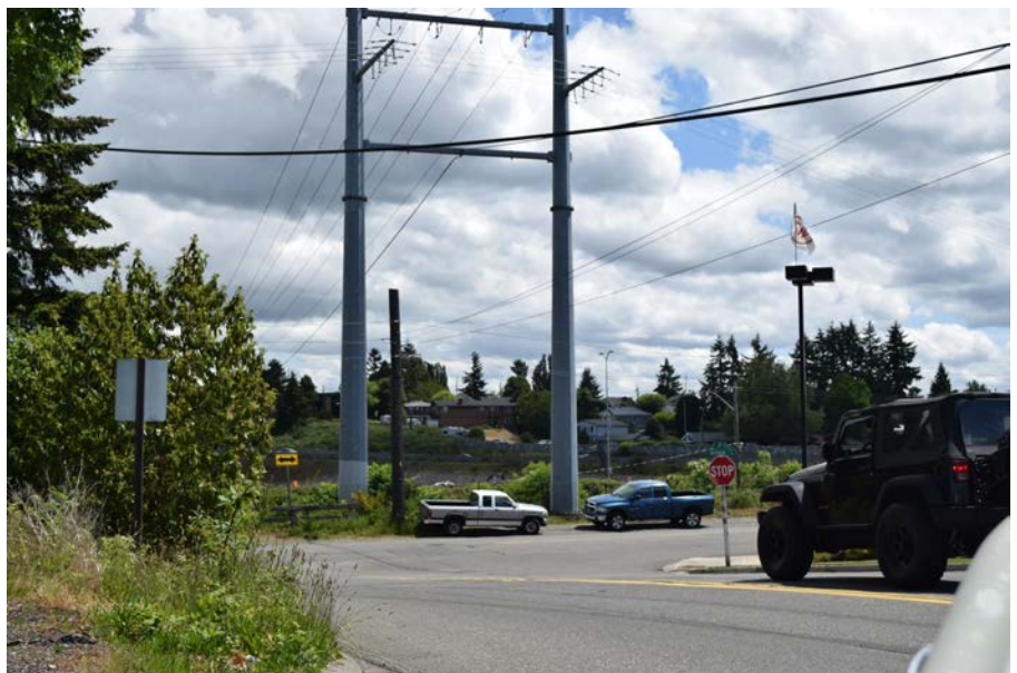
Photo US-3. Overhead powerlines, S. Sprague Ave.
