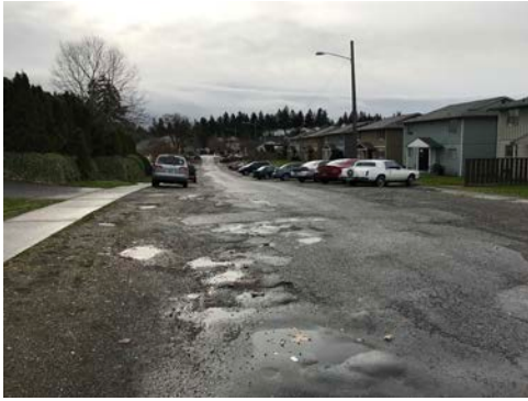
Photo T-10. Multiple streets in the area require maintenance.
